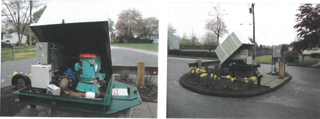
Figure 4 - Plaza Street Pump Station
