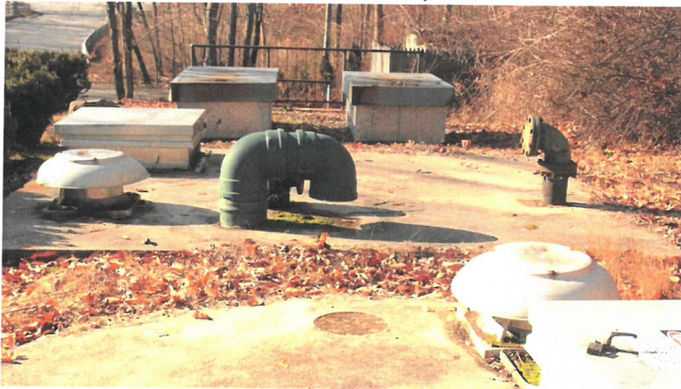
Figure 3 - Tatnic Road Pump Station
