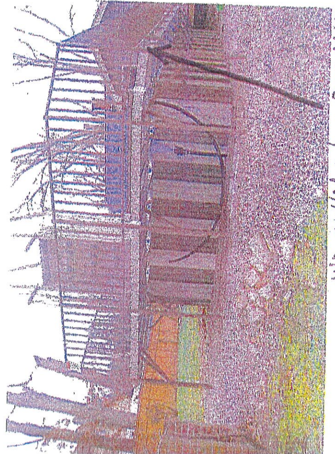
We pulled a tape from this point of the deck to the existing garage.
