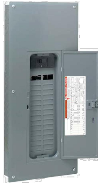
PHOTOVOLTAIC AC DISCONNECT NEC 690.54
