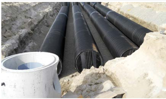
CDS pretreats a rainwater harvesting cistern.
