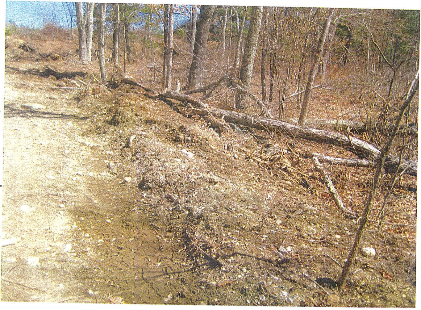
Road widened near stream crossing showing fill deposited in Upland Review Area.
