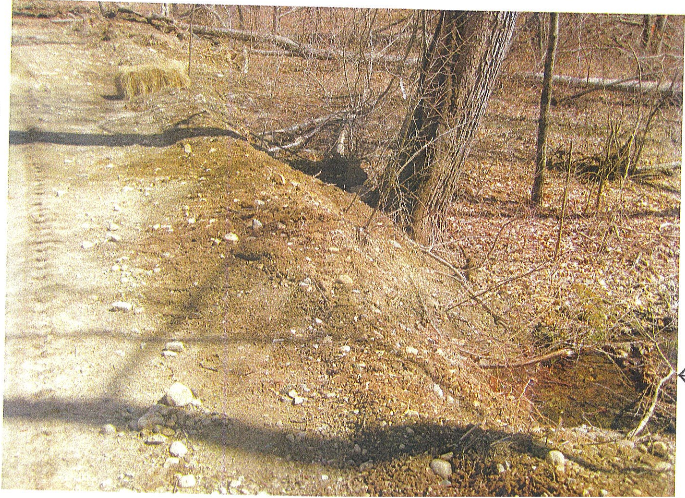
Fill pushed into wetlands to widen road at existing stream crossing.
